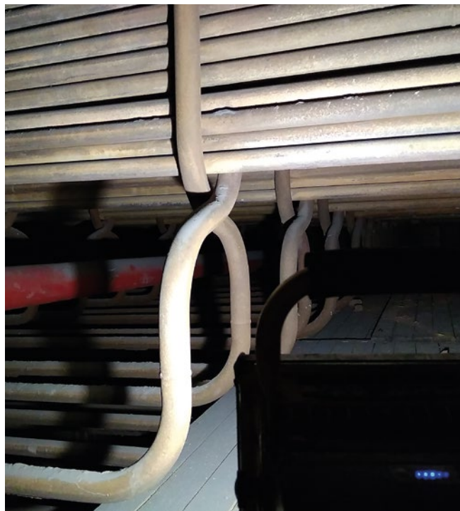
View of the internal part of the boiler after the installation of soot blowers
