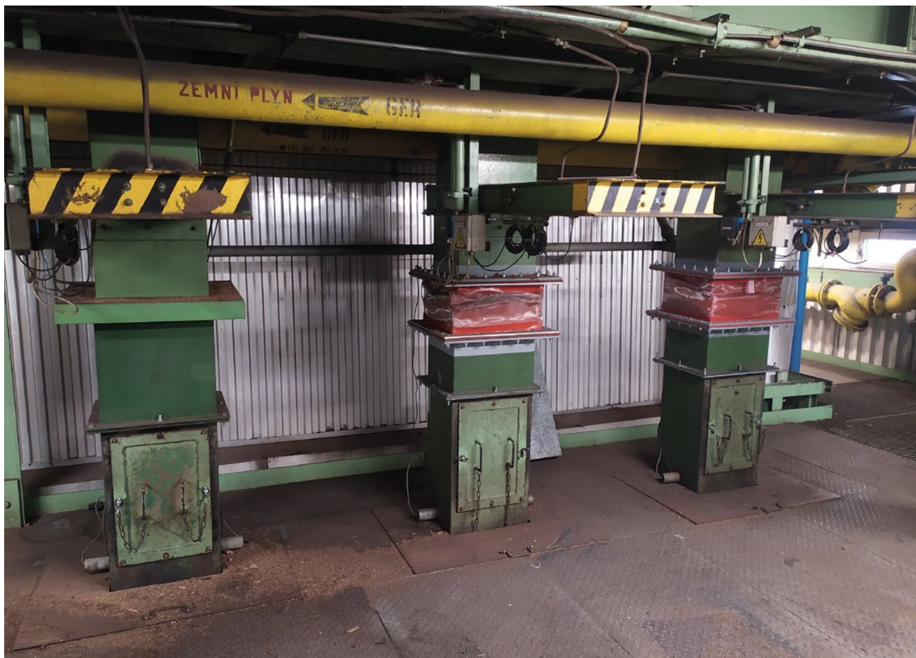
Supply and replacement of a metal expansion joint with a fabric one, flange type, including steel components (in the centre and on the right)
