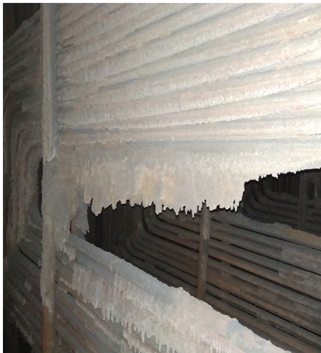
View of the internal part of the boiler before the installation of soot blowers
