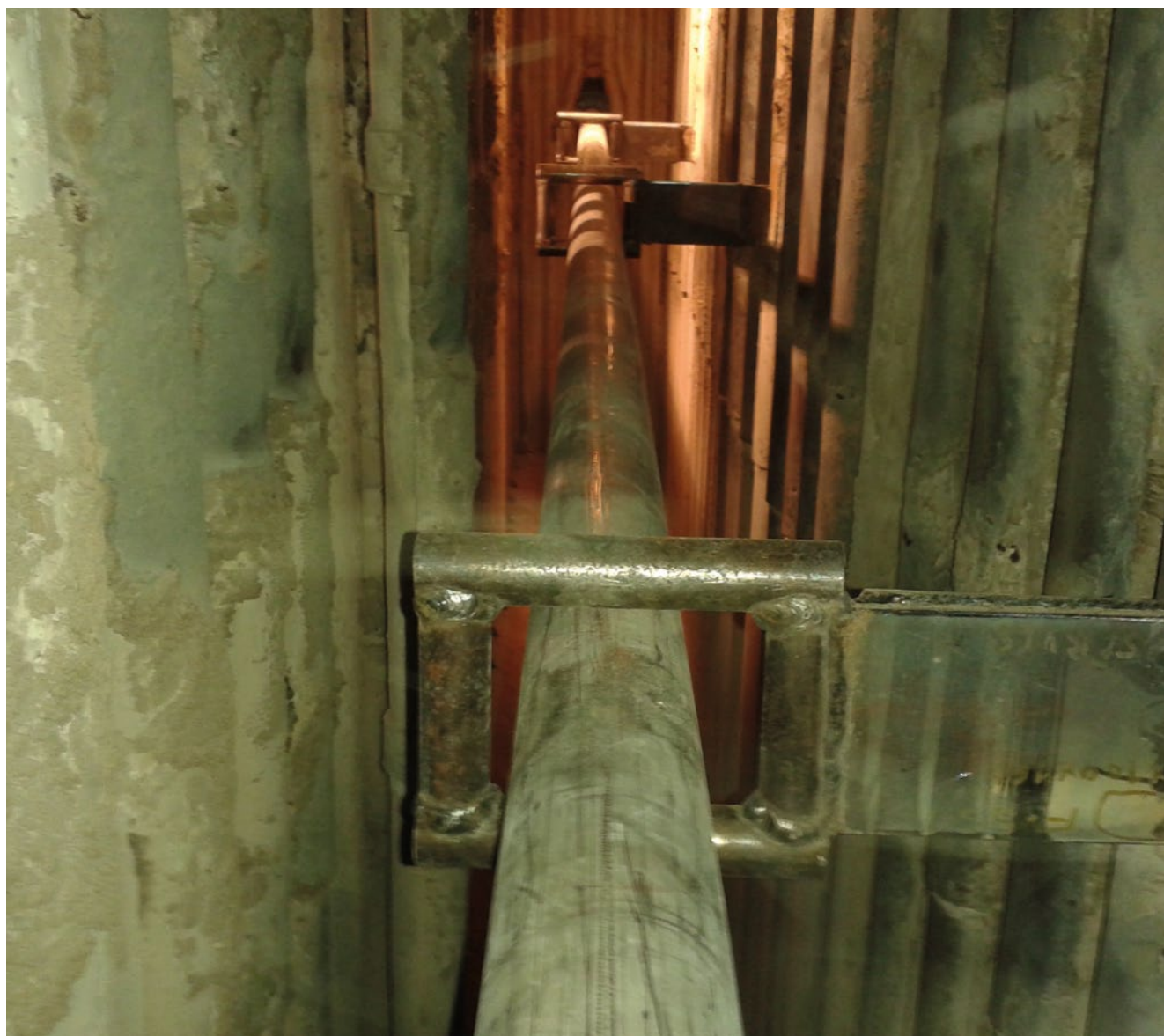
Repair of the soot blowing pipe in the internal part of the boiler
