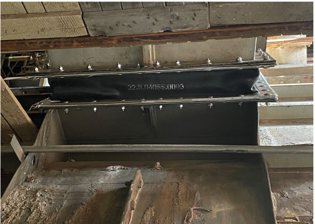
Supply and replacement of a broken rubber expansion joint with a new one, including pressure flanges
